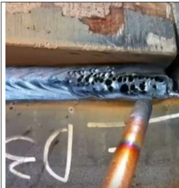
Defektan, porozan var
